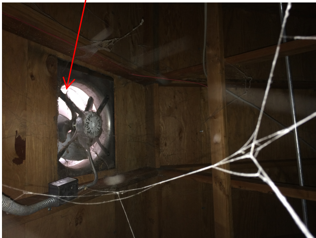
existing vents - supply air not sufficient
