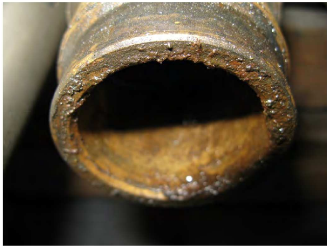
Picture #8 The oil tube bearing is worn and will be replaced.
