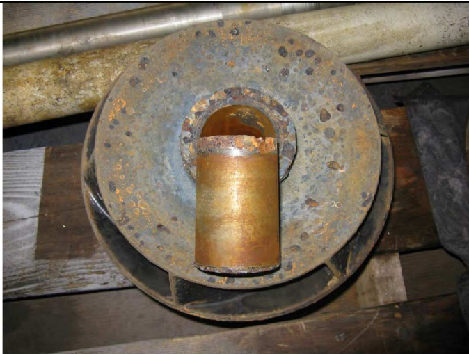
Picture #14 Impeller and collet. Impeller to be reused with the collet being replaced.
