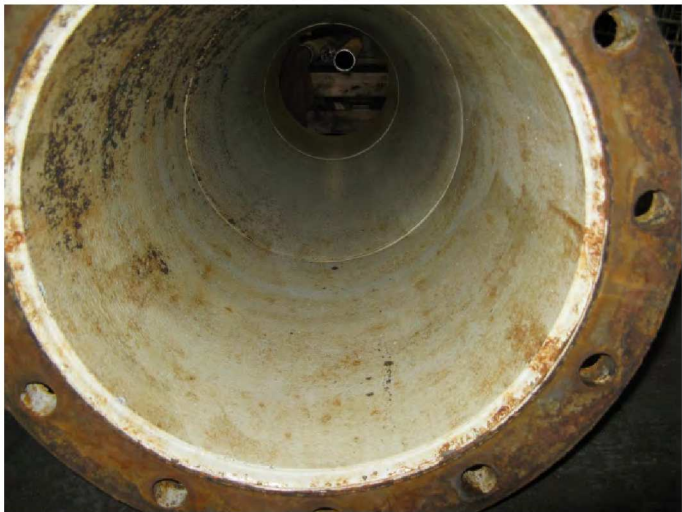
Picture #9 Trans-cone ID . Recommend blast and recoat.
