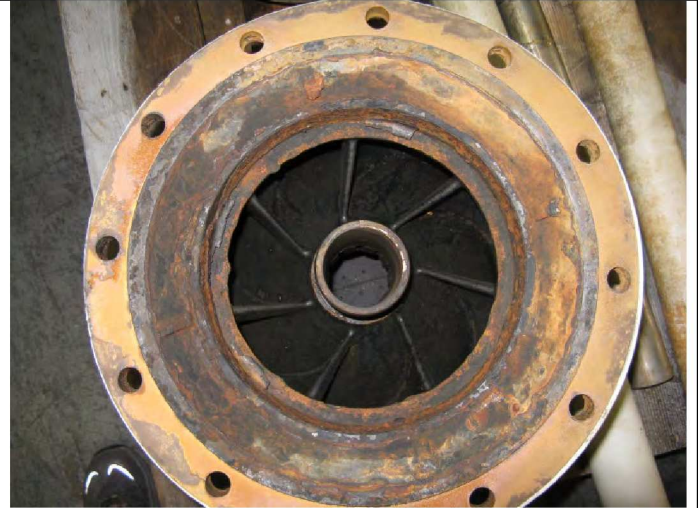
Picture #13 Bowl showing herisite lining. Flanges will be power wire brushed prior to reassembly.
