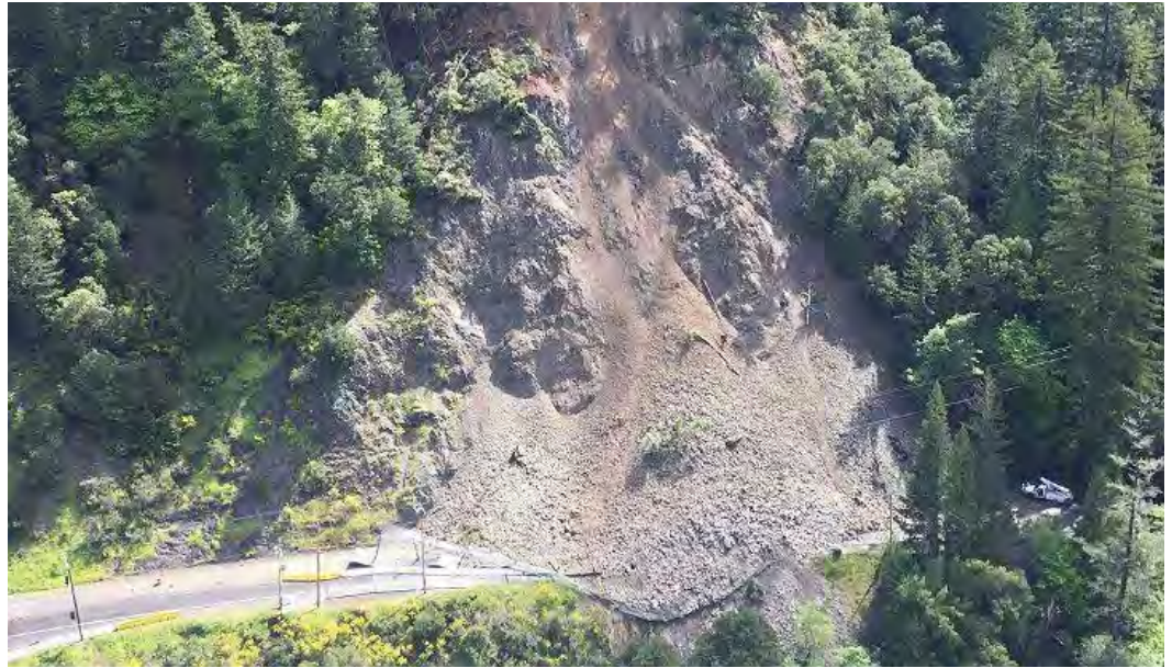
Figure 4-43: Landslide on Highway 101
