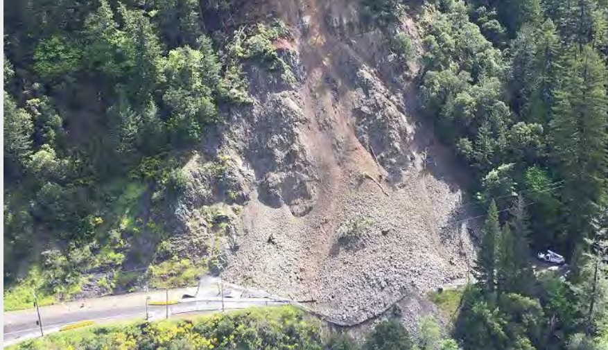
Photo shows a 2017 landslide on Hwy 101 near Leggett, https://sanfrancisco.cbslocal.com/2017/04/20/massive-landslide-shuts-down-highway-101-in-mendocino-county/
