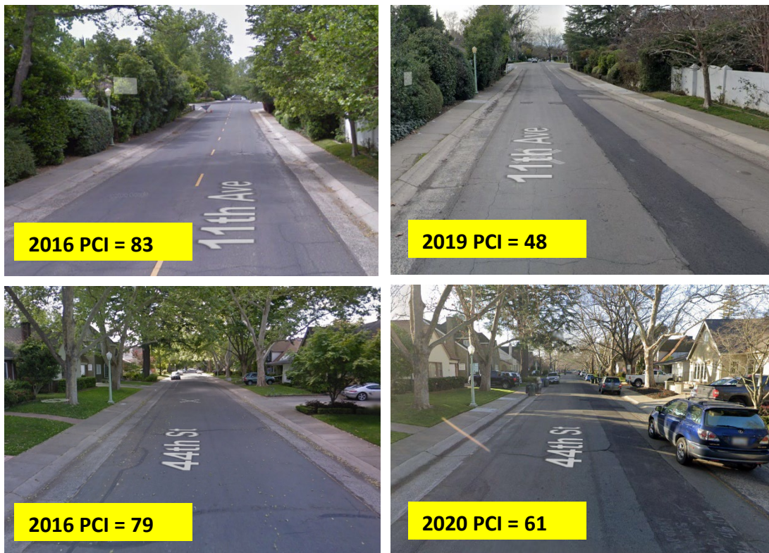
Figure 2. Comparison of Pavement Condition With and Without Utility Cuts
