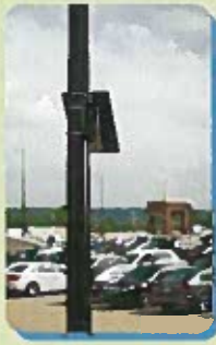
Solar & Existing Pole
