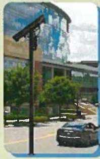
Solar & Flock Pole
