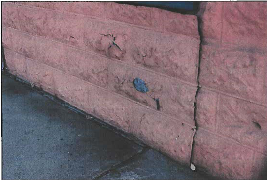
Photo 37: West elevation, condition of pressed tin
