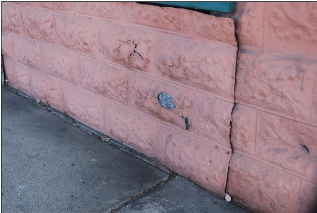
Photo 36: West elevation, condition of pressed tin
