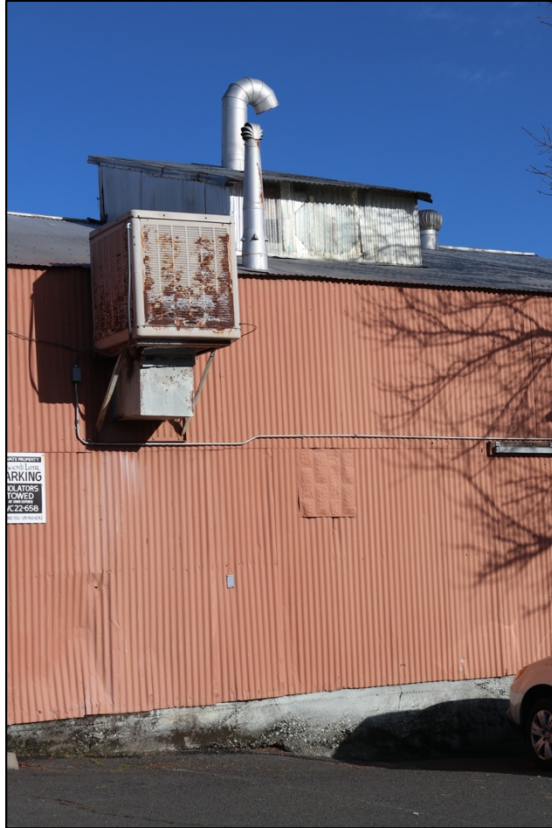
Photo 41: South elevation, mechanical equipment detail
