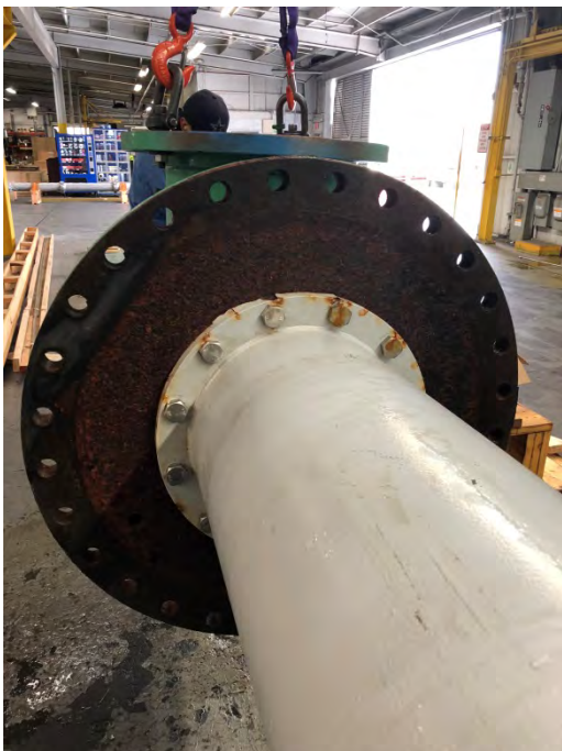
Picture #8 – Rust on the back side of the discharge will be removed prior to reconditioning
