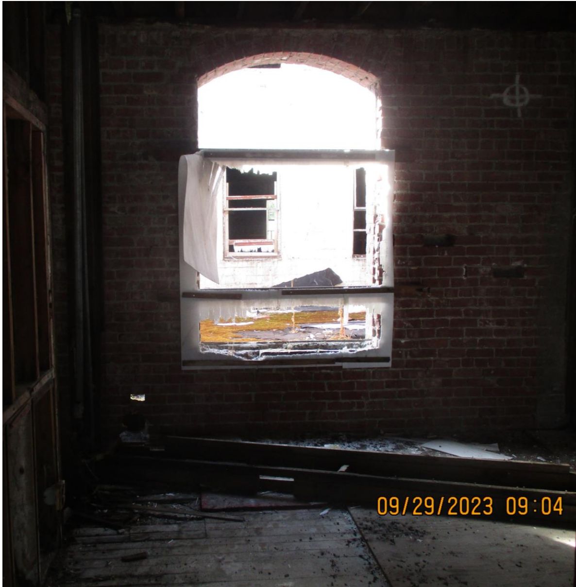
2 ND FLOOR LOOKING AT WEATHER PROOFING FAILURE
