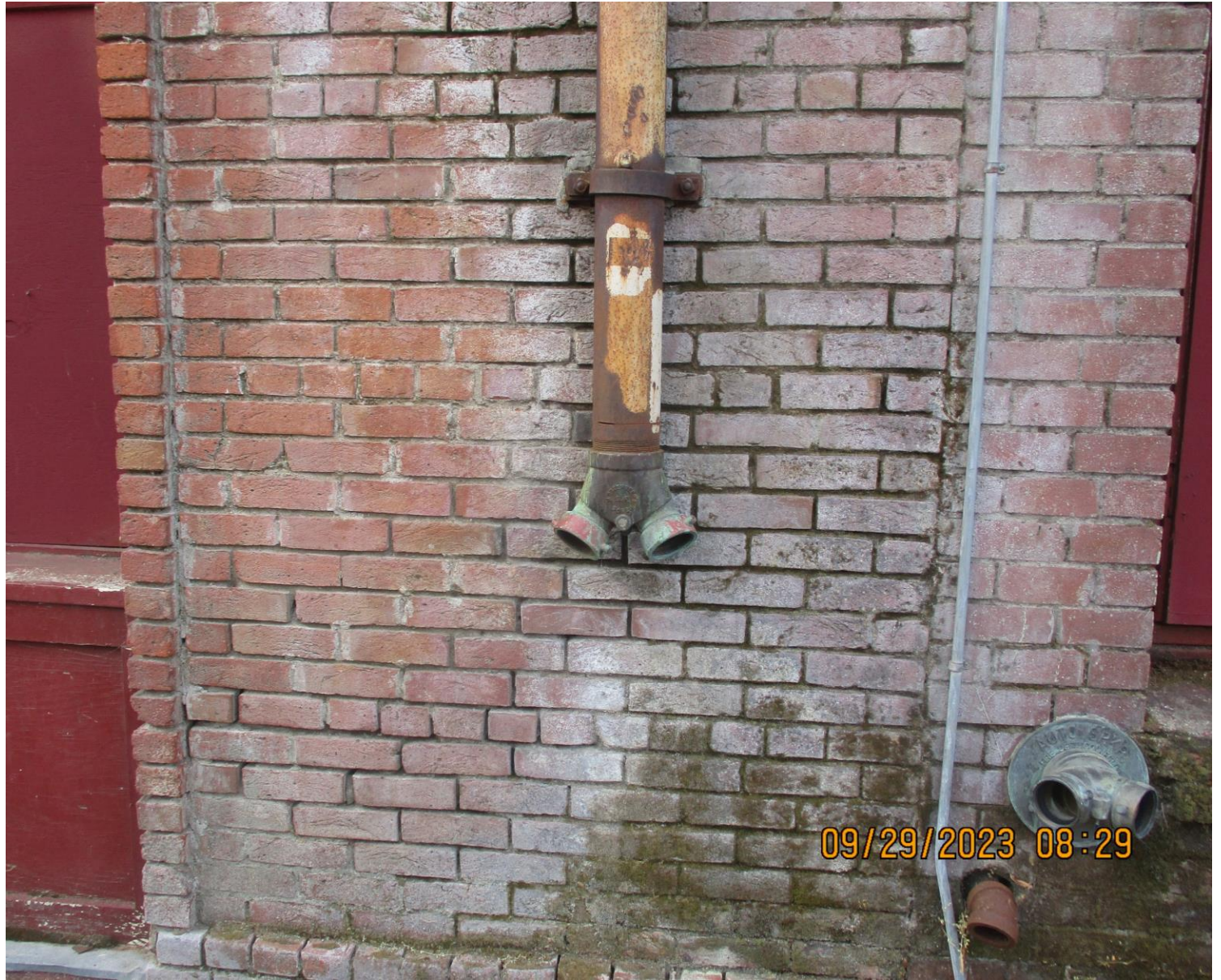
SMITH ST FDC AND STANDPIPE
