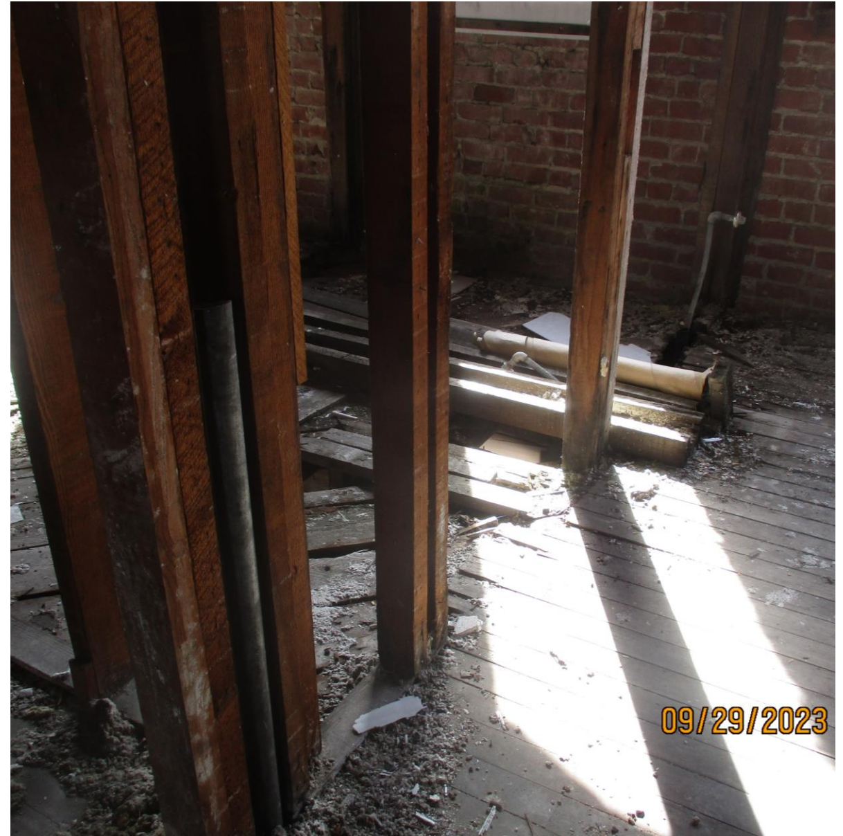
STRUCTURALLY COMPROMISED FLOOR
