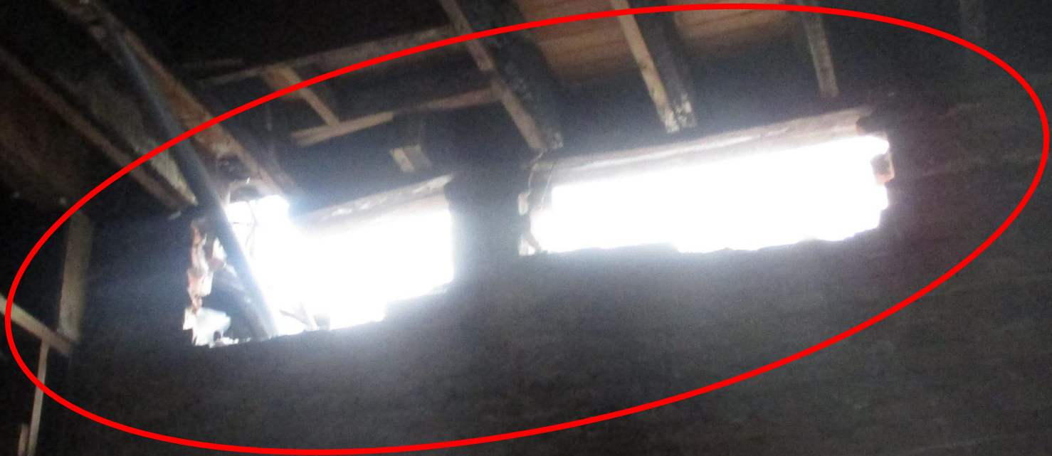
1 ST FLOOR BRICK WALL STRUCTURAL FAILURE
