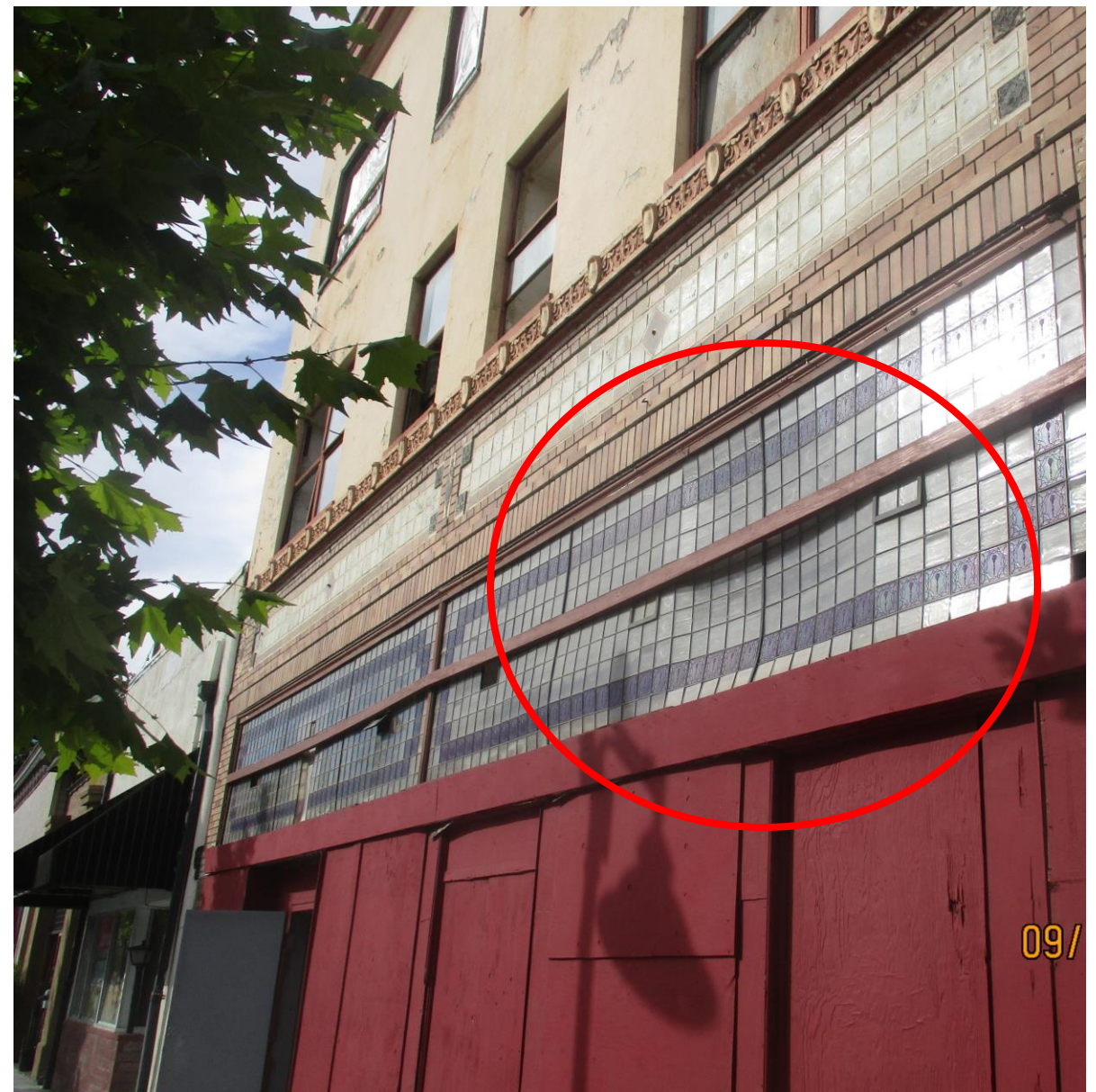
LEAD GLASS FAILURE STATE ST
