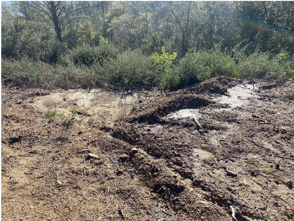
Photo 2. Location 2: Road conditions after rain.
