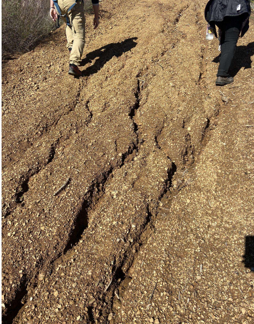
Photo 14. Location 11: Severe water damage to road.
