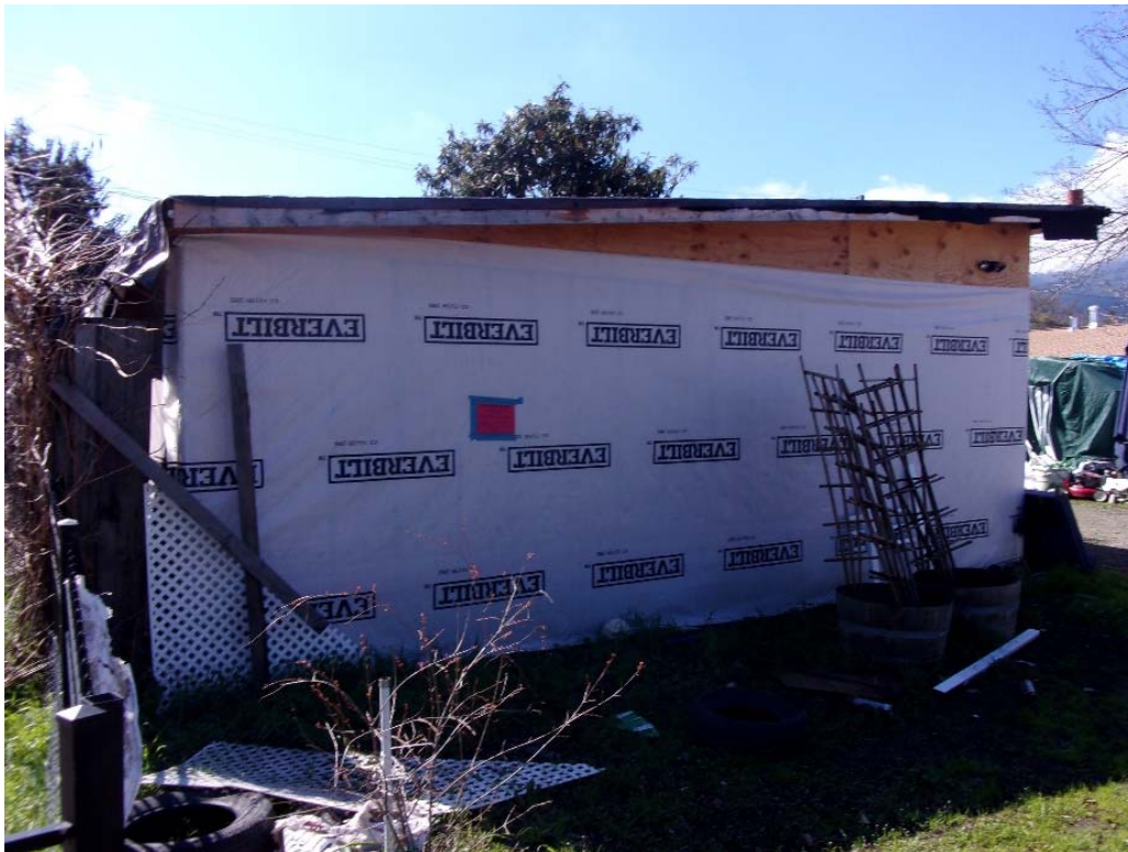
Code violations and illegal structures, posing unsafe environment.
