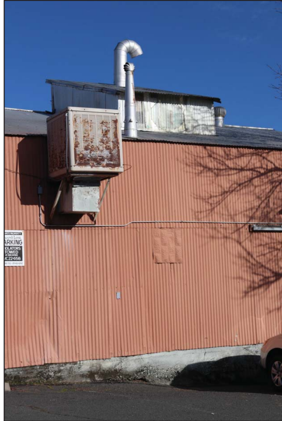
Photo 41: South elevation, mechanical equipment detail
