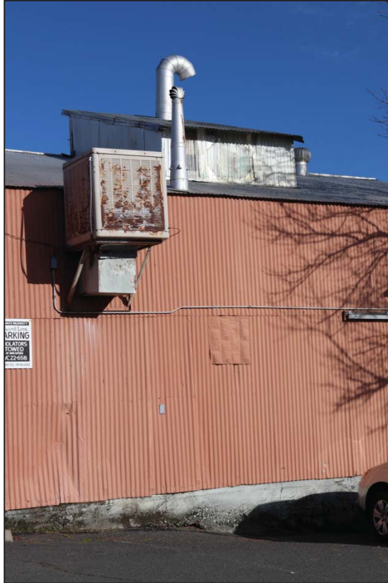
Photo 41: South elevation, mechanical equipment detail
