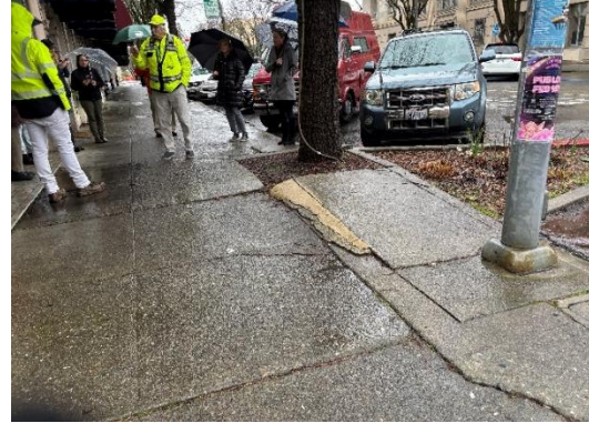
Tree roots impacting utilities, drainage, and sidewalk on School Street.
