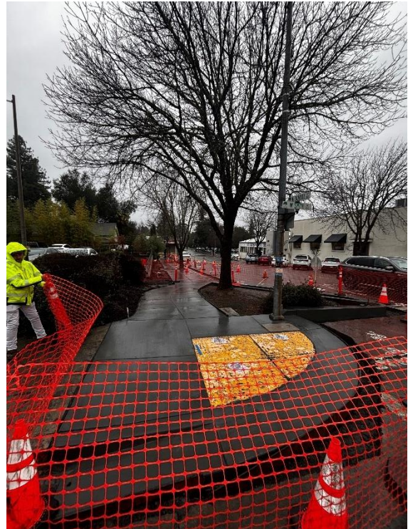
Recent reconstruction of the northwest corner of the School Street and Smith Street Intersection.
