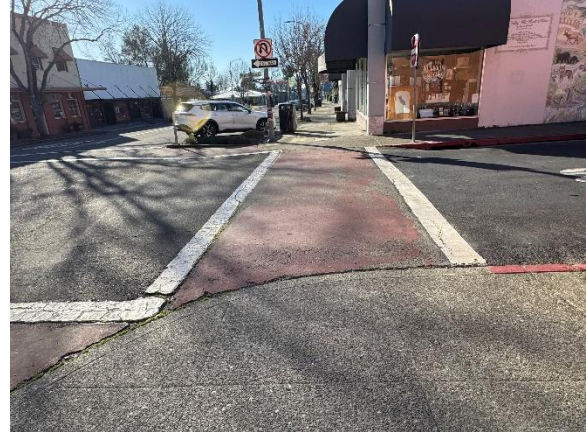
Faded crosswalk and lack of ADA curb ramps on the west leg of Church Street.
