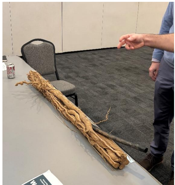
Tree roots wrapped around a water line, found at School Street and Smith Street.
