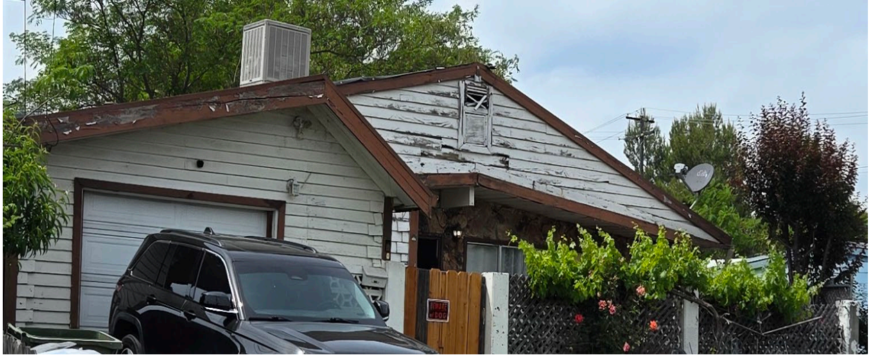
Example: Housing Unit in a Condition of Moderate Deterioration
