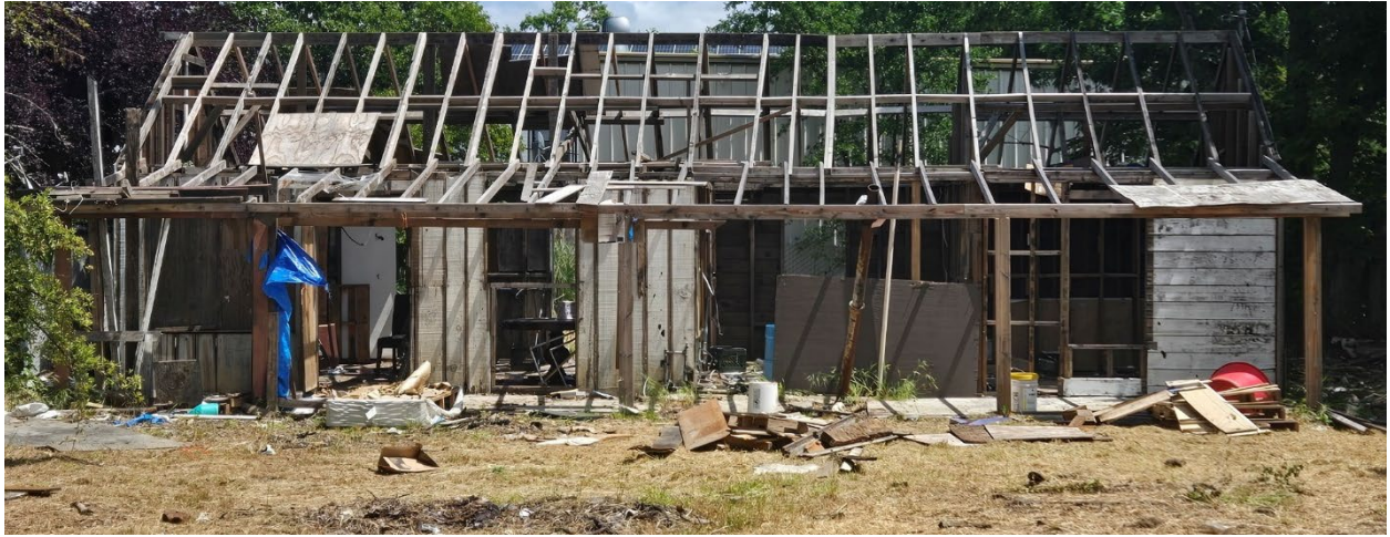
Example: Housing Unit in Dilapidated Condition
