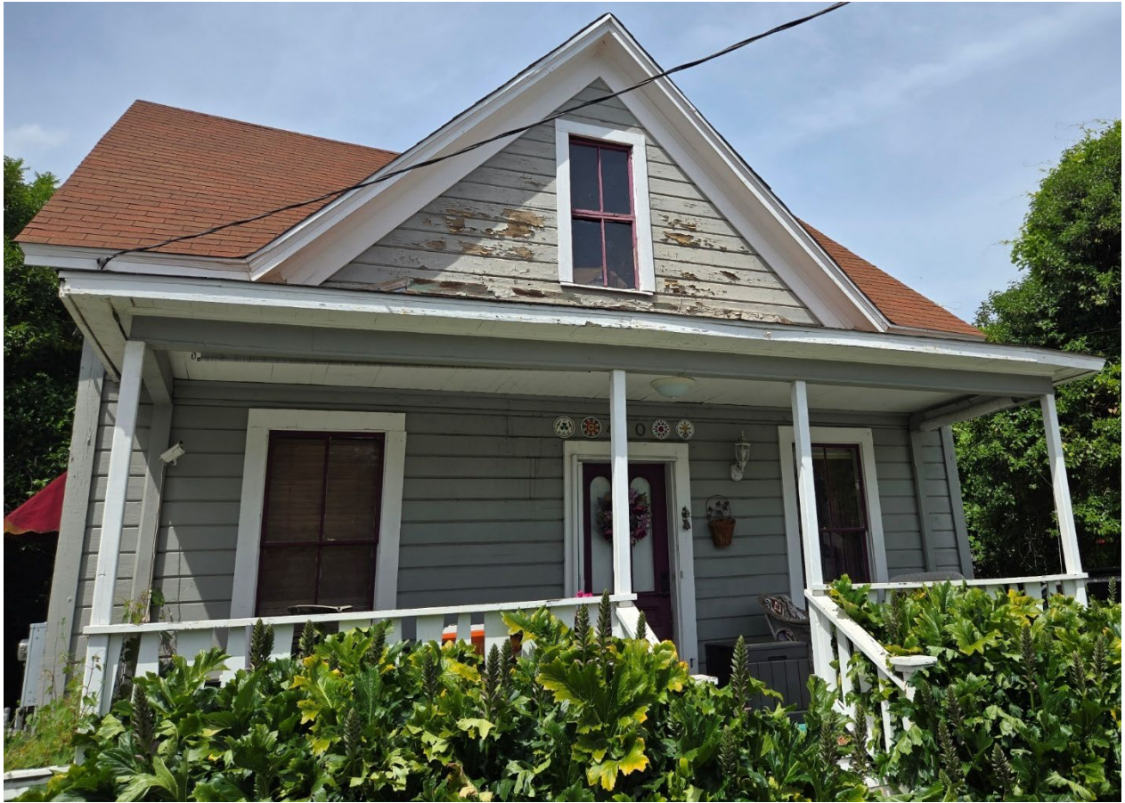
Example: Housing Unit in a Condition of Minor Deterioration
